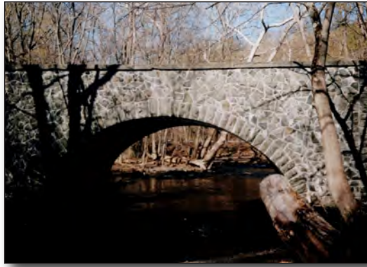
Above: Photo of bridge over Black Creek just south of the Black Creek Apartments, shown below. Designed and built by Julian Burroughs.
